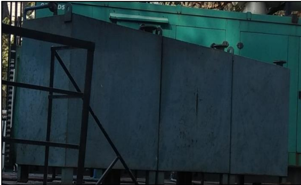
Diesel storage tank for DG set
