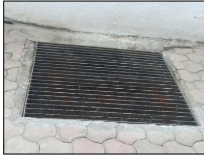
Rain water harvesting system
